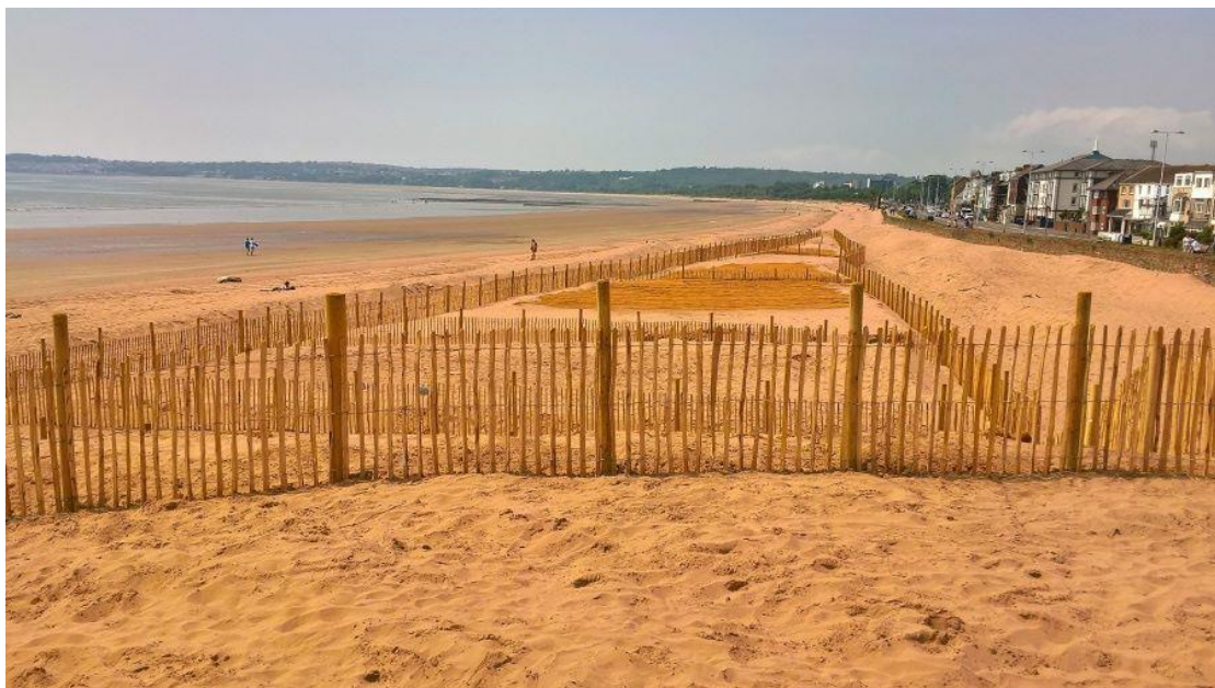
Figure 3 Installation of fencing and use of geo textile matting to trap sand at Swansea Bay
