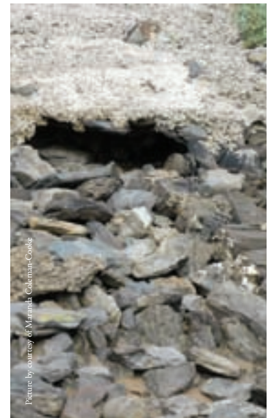
TIDES ERODE BENEATH MODERN CONCRETE REPAIRS
