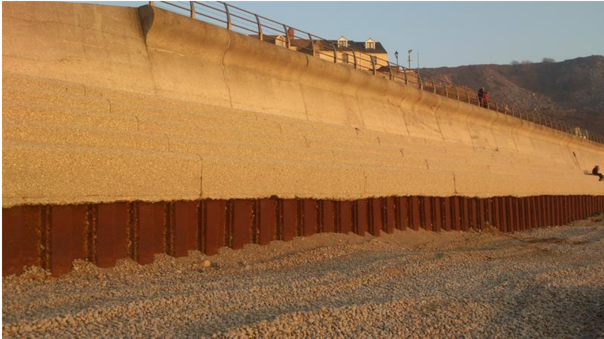
Figure 23 - Flood defence sea wall on Chesil Cove Beach, Dorset (BennH, 2014, https://commons.wikimedia.org/wiki/File:Chesil_Cove_flood_defences.png [unedited]).
